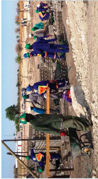
PRIORITY AT MCA-N CONSTRUCTION SITES: HEALTH AND SAFETY GEAR FOR THE WORKERS
