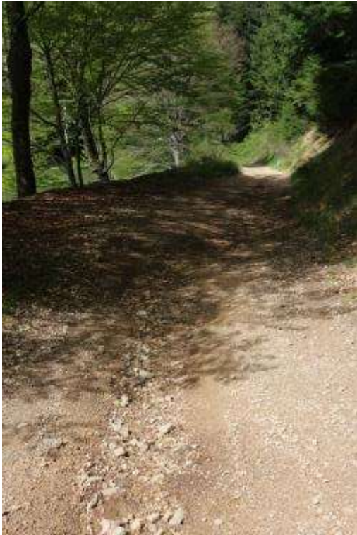
Figure 22: Ornières larges en forte pente
