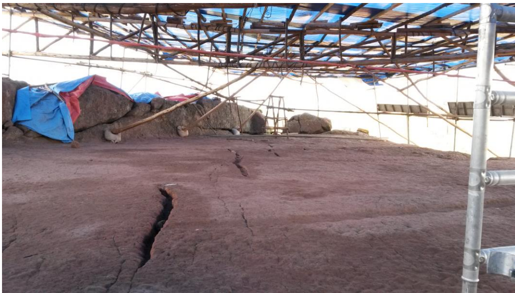
Fig. 2.3. The natural crack on Bete Gabriel's roof
