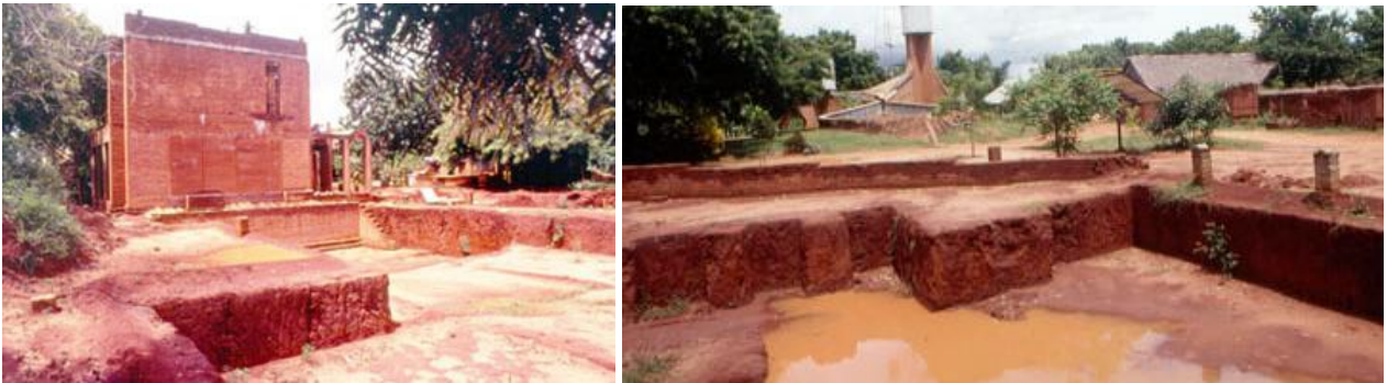
Figure 65 ( Left & Right) Excavation of the basement floor – 1.2 m below ground level. Source: (Auroville Earth Institute , Undated)
