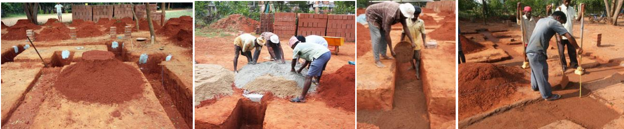
Figure 68 (Left 1) Soil sieved from the digging trench. Source: (Auroville Earth Institute , Undated)
