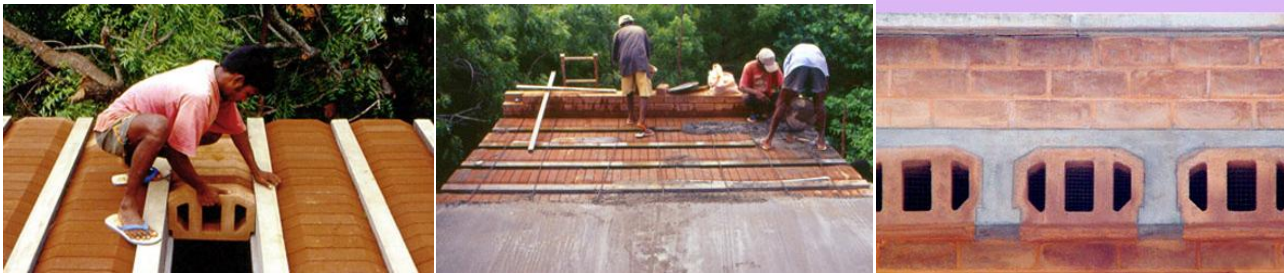
Figure 75 (Left) Adjusting Hourdi blocks on T beams. Source: (Auroville Earth Institute , Undated)
