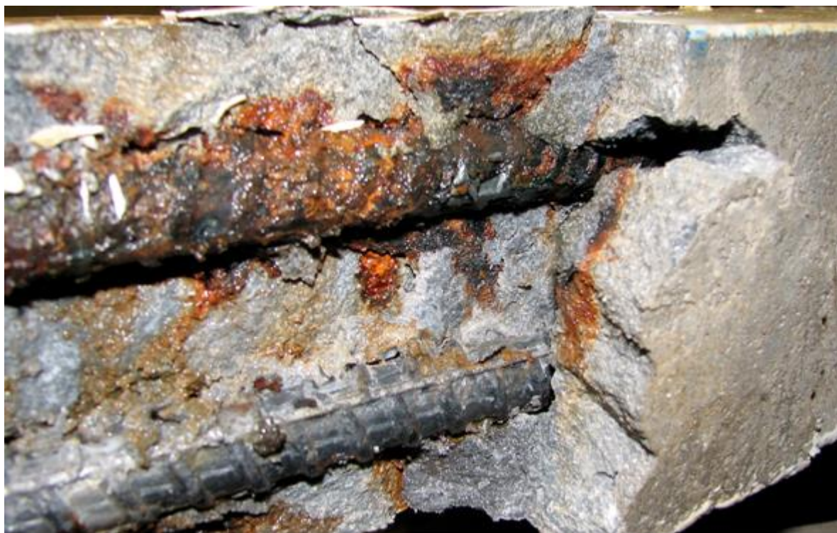
Figure 1-3: Corrosion des armatures
