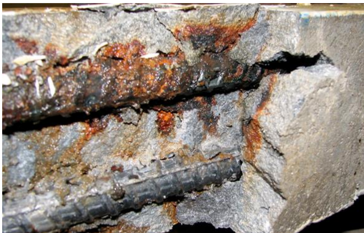
Figure 1-3: Corrosion des armatures
