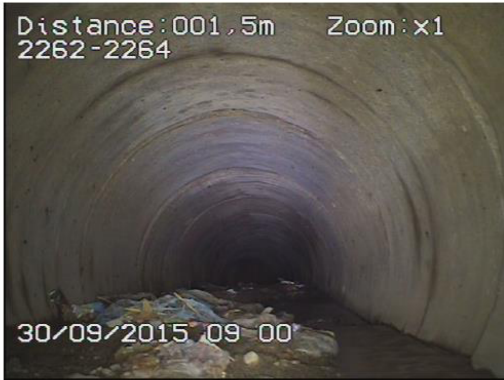
Figure 35 : Photo N°2262_0760 issues des inspections hydrozoom
