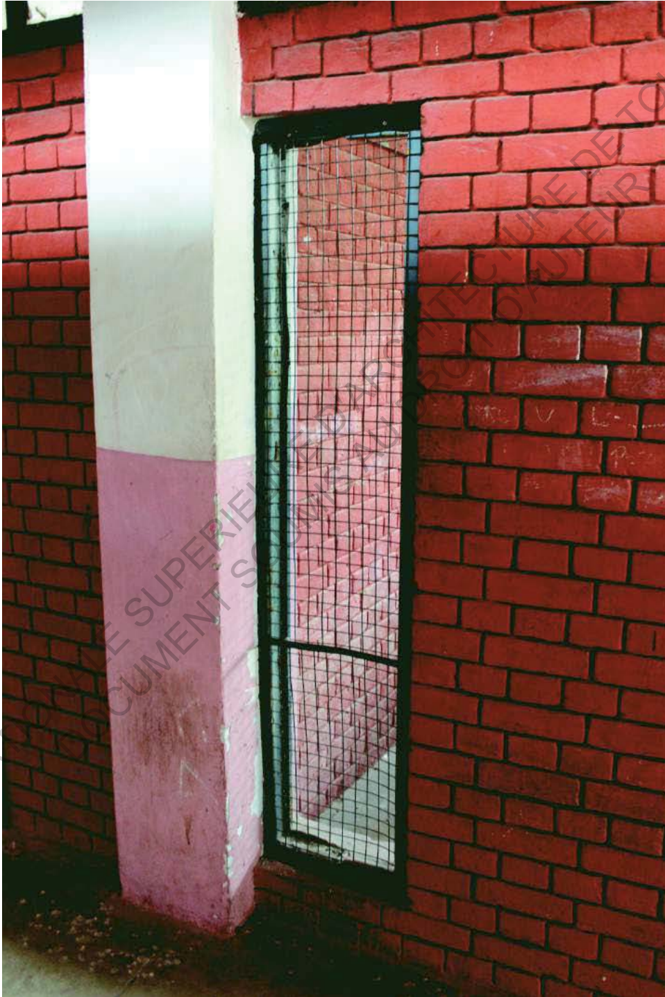
Grille de ventilation – Secondary School S.22 – Image personnelle
