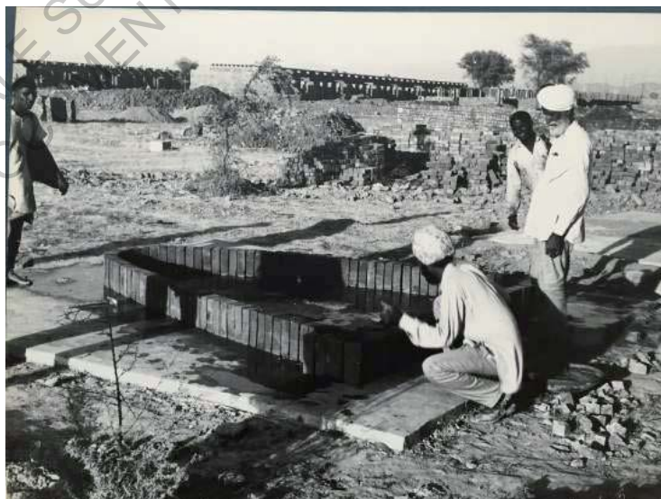
Fond d'archives du Canadian College of Architecture de Montréal, photographie « During the construction of the Higher Secondary School, Sector 22, 1953 »
