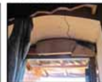
Absence d'un linteau Pudaenior modi is mo
