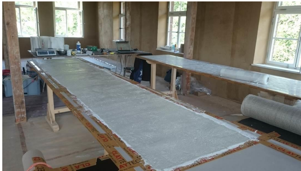
Joints between work surfaces covered with cardboard but still showed through
