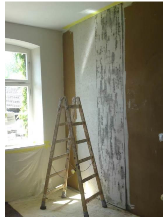
The very same piece of wallpaper stuck to a new umbra paint base
