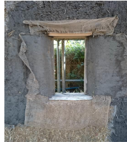
Loadbearing strawbale building site in Romsey, UK: Window reveals in straw wall receive bonding coat, then body coat, then jute mesh and then finishing coat.
