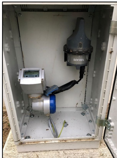
Fig. 5. Data Logger SOFREL LS42
