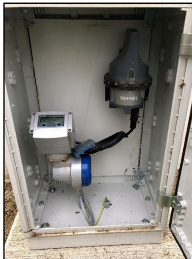
Fig. 5. Data Logger SOFREL LS42
