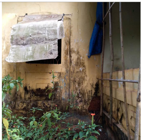
Maintenance and repairs: A make-shift overhang covers the window on the front facade.
