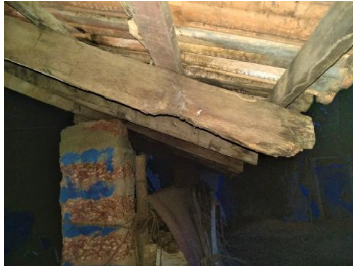
The last baton along the edge of the roof is placed with the smaller side resting on the rafters. Image 124 and Image 125: (Survey no. 8). Image 126: (Survey no. 3a).
