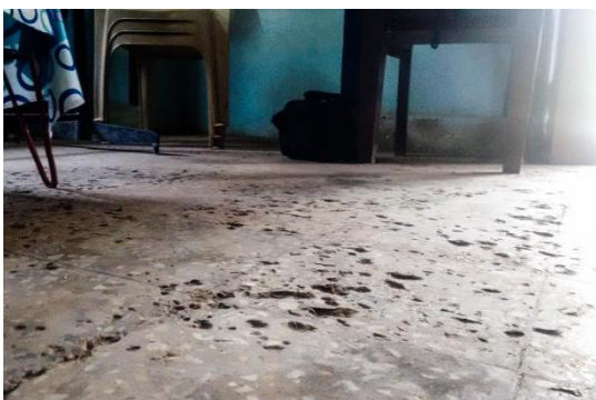
Damages incurred / problems faced: Chip-tiles are chipped-off.
