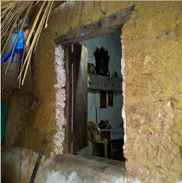
Plasters: Thin coat of lime on earthen walls (interior), including window jambs.
