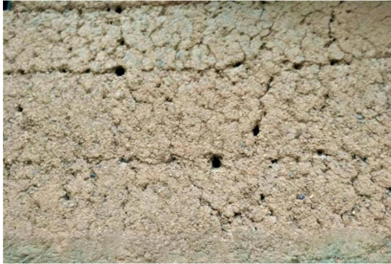
Image 70: Holes along the horizontal 'lift' joints, which perhaps indicates the use of form-work in cob construction (Survey no. 11).
