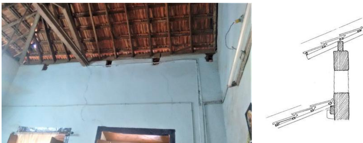
Image 98: Vents along wall tops (Survey no. 3a). Image 99: Section of a vent (Survey no. 11).
