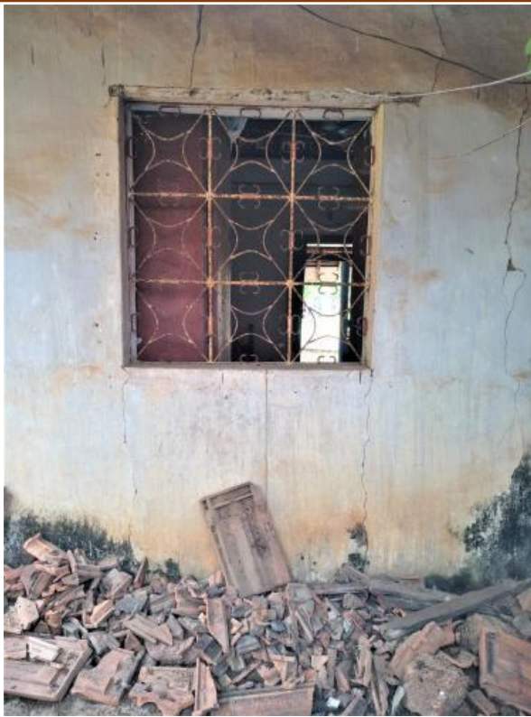
Image 138: The lack of support provided by rotting lintels caused the roof to put pressure on the wall, and created many cracks around the window (Survey no. 7).
