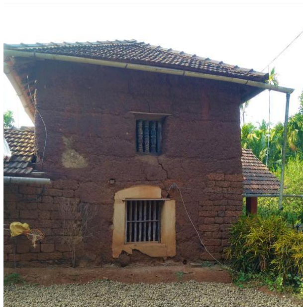
Image 76: Corners; lower walls in laterite masonry, upper walls in earth. Some parts of the walls were also built in laterite masonry. (Survey no. 15)
