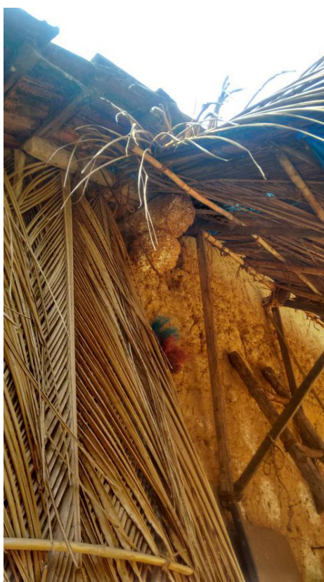
Image 123: Two decoratively cut laterite-stones that jutted-out from the wall top were probably meant to support the roof framework, but sometimes aided in holding the overhangs as well. (Survey no. 1).
