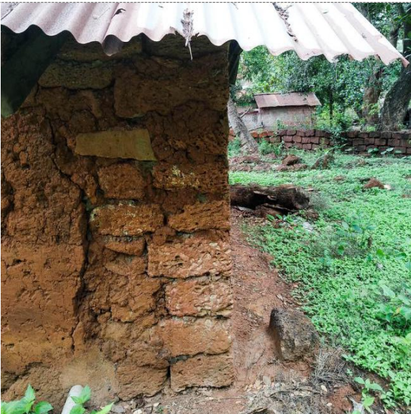
Observations: The laterite masonry in the corners has earthen or cement mortars. It is hard to say whether these corners are part of the original construction or a later addition.
