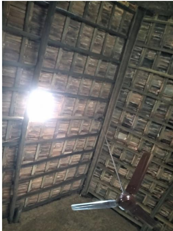
Image 115: The ridge of the roof framework was made from the trunk of the coconut tree. The trunk was split into two and the fibre from its core was taken out, forming a hollow in the middle. (Survey no. 6).
