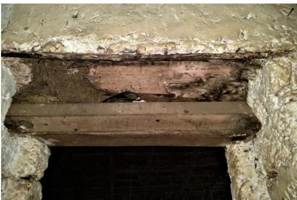
Damages incurred / problems faced: Rotting of lintels.
