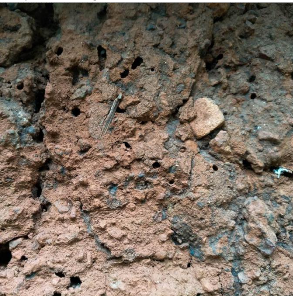
Damages incurred / problems faced: Mason-bee holes
