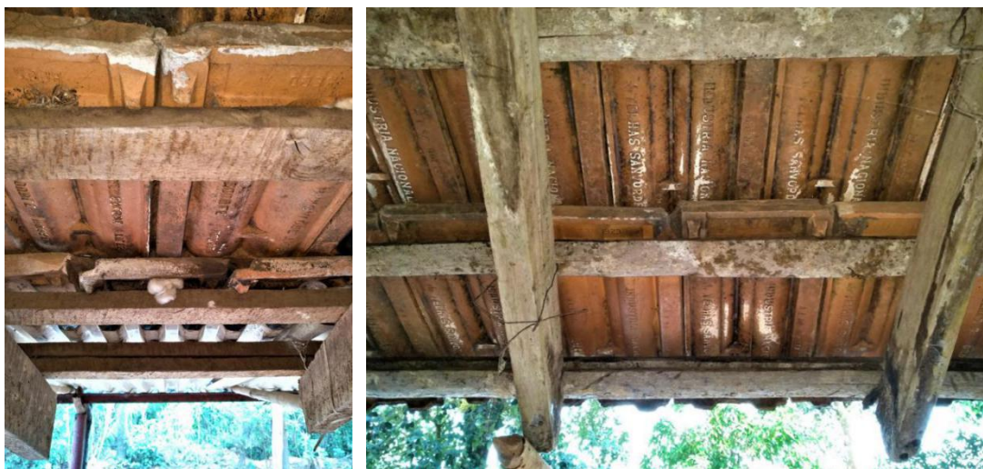
Image 127: Two, instead of one baton was fixed along the ends of the roof's framework (Survey no. 13). Image 128: Splits of the beetle-nut tree were used as batons. Two batons were used along the roof-line. (Survey no. 12).
