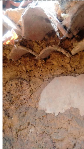
Damages incurred / problems faced: Mason-bee holes on the repaired part.
