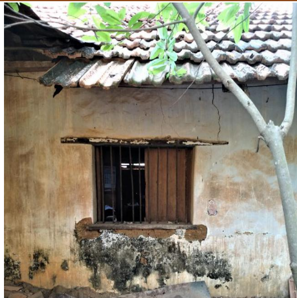
Damages incurred / problems faced: Cracks, especially near lintels.
