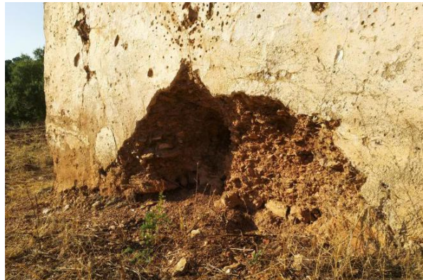
Damages incurred / problems faced: Holes in walls especially where there is lime-based plaster.
