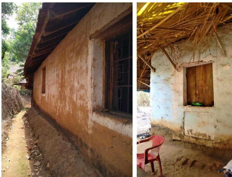
Image 87: A small, earthen gradient covered the foot of external walls (Survey no. 12).
