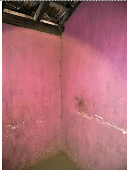
Damages incurred / problems faced: A crack appeared just after the construction was complete.
