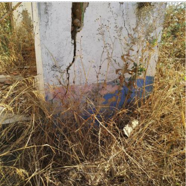
Damages incurred / problems faced: Cracks appeared and the walls began falling apart.
