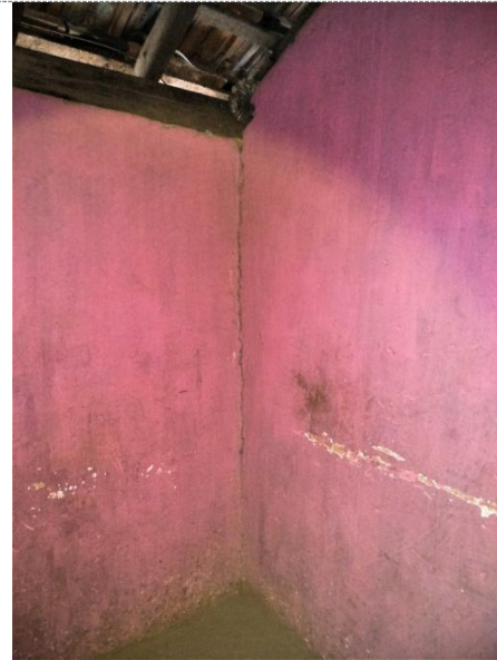
Damages incurred / problems faced: A crack appeared just after the construction was complete.
