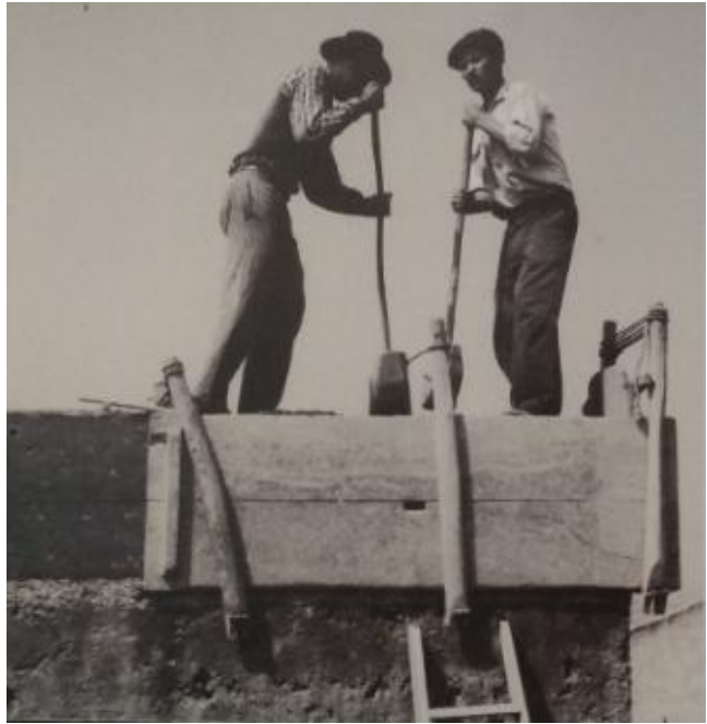
Traditional rammed-earth form-work used Aldeia da Luz in Évora before the 1950's. [Source: Panel at Museu da Luz, Luz, Évora, 2018]
