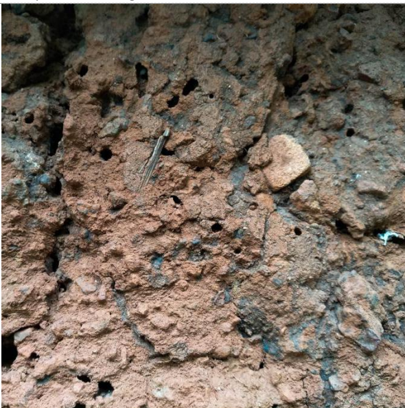
Damages incurred / problems faced: Mason-bee holes
