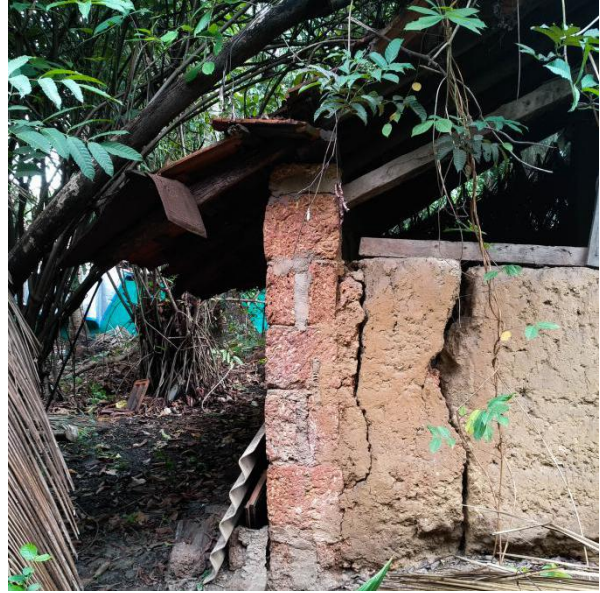
Damages incurred / problems faced: Structural cracks.
