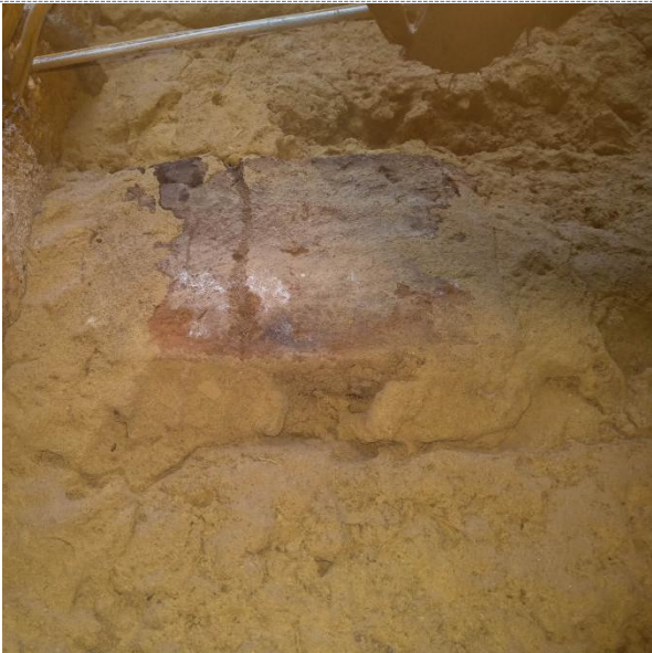
Observations: There is a (piece of) fired brick in the adobe-brick gable.
