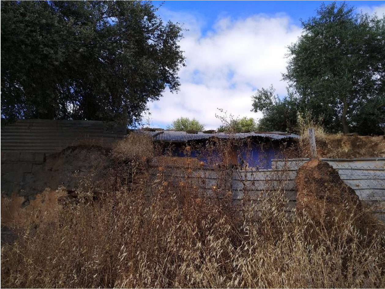
A partly-collapsed building exposing an internal walls of an old, 'Taipa' house. Blue pigment paint seen. (Picture taken in July and August 2018)
