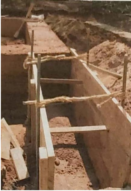
Form-work with ribs and spacers ('kani' in Konkani) [Source: Lobo, Earth in Architecture , 2006, p.42]
