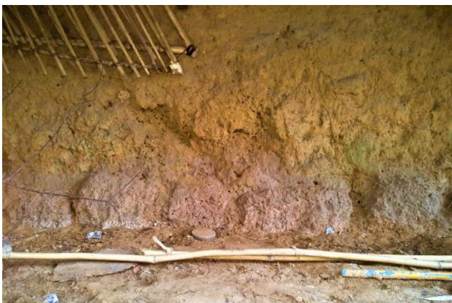
Damages incurred / problems faced: Erosion of the walls has created depressions above base-courses of external walls.
