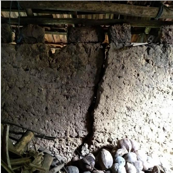
Damages incurred / problems faced: Structural cracks.
