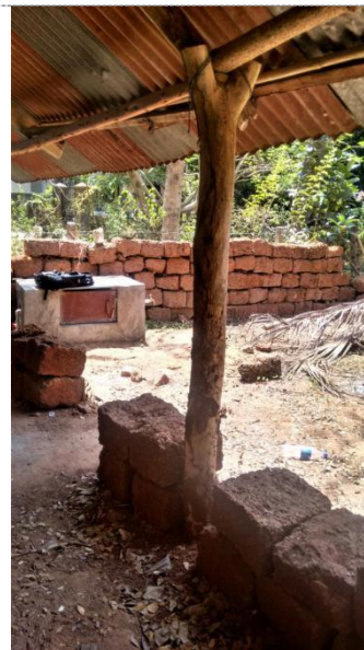
Observations: A make-shift lean-to aids in protecting facade walls from rain water. Simple branches are used to support the roof of the lean-to.
