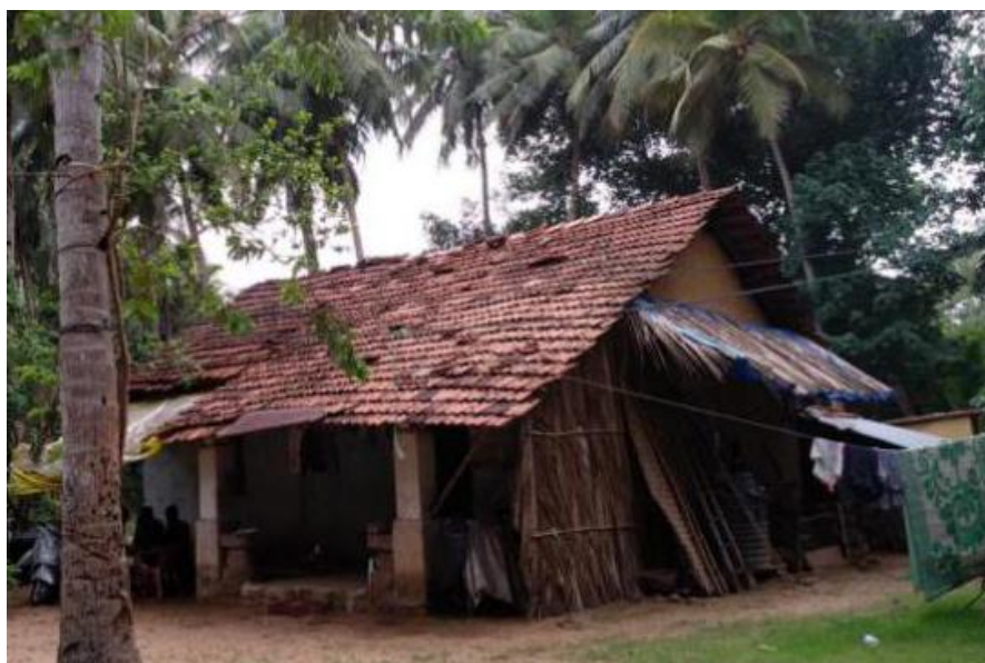
Image 133: Palm-leaf barriers poised parallel to earthen walls protected the walls from rainwater (Survey no. 1).
