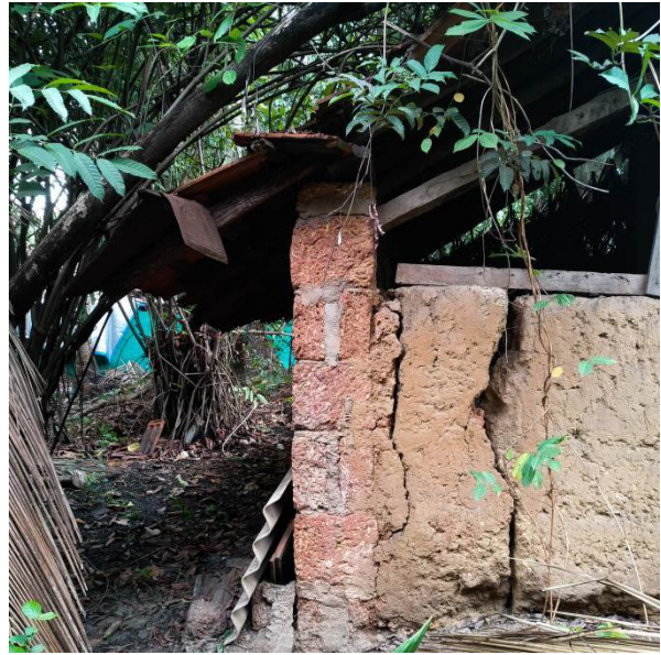
Damages incurred / problems faced: Structural cracks.
