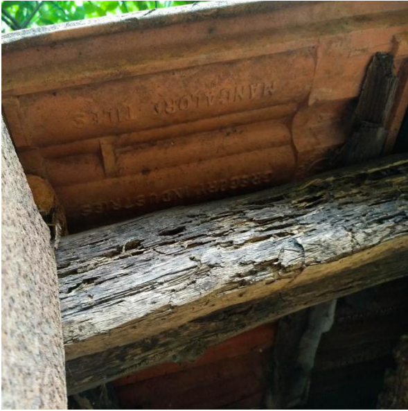
Damages incurred / problems faced: Roof-frame is rotting.
