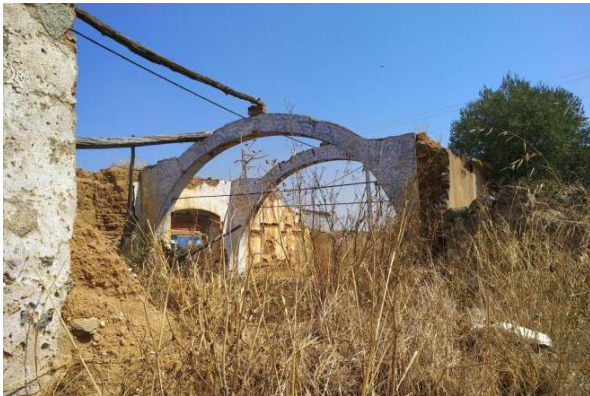
Distinct architectural details: Arches on the interior. Maintenance and repairs: Ties between arches.
