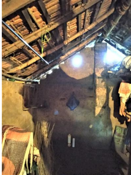
Image 117: Sometimes, bamboo and other similar materials were used even in the case of 'Mangalore-tiles' roof framework as well (Survey no. 4).
