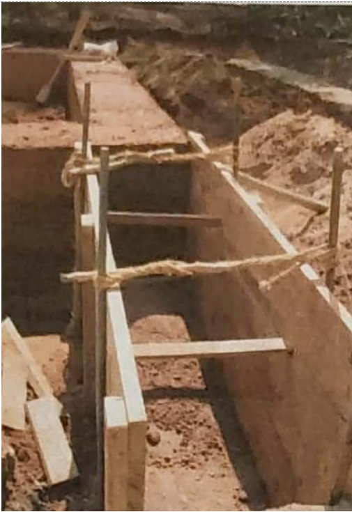
Banche traditionnelle et entretoise ('kani' in Konkani) [Source: Lobo, Earth in Architecture , 2006, p.42]
