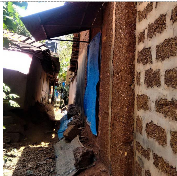
Maintenance and repairs: Overhangs over facade windows protect interiors from rainwater. The gradient and window along the north are covered with Tarpaulin.
