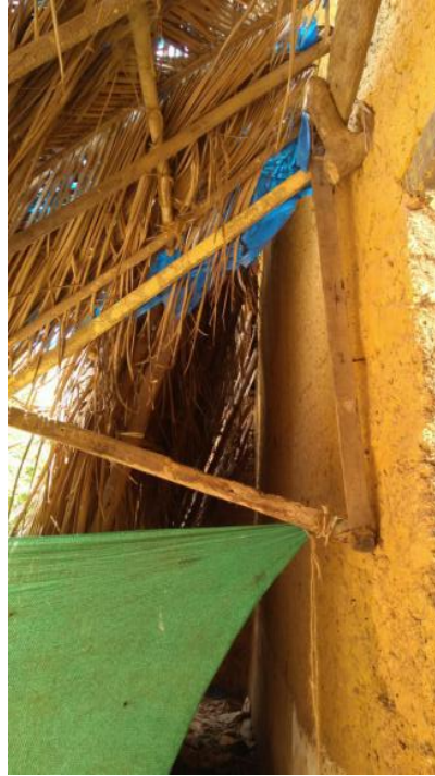
Image 122: In Survey no. 8, make shift hooks were observed.
