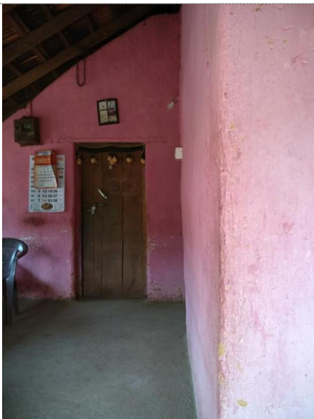
Damages incurred / problems faced: Bulging of wall.
