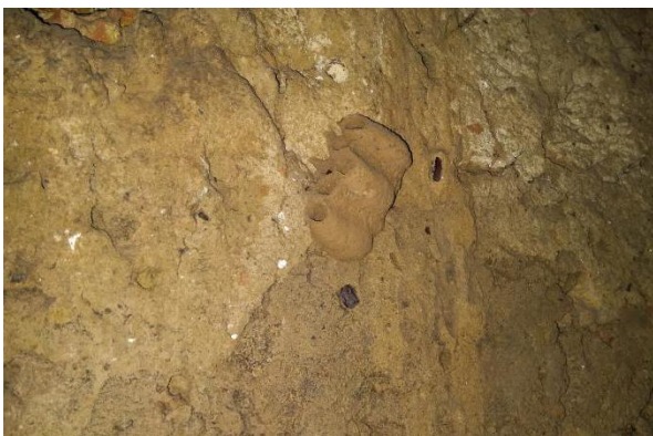
Damages incurred / problems faced: Honey-bees build earthen-nests on the wall surfaces, and store worms in them, especially during the monsoons.
