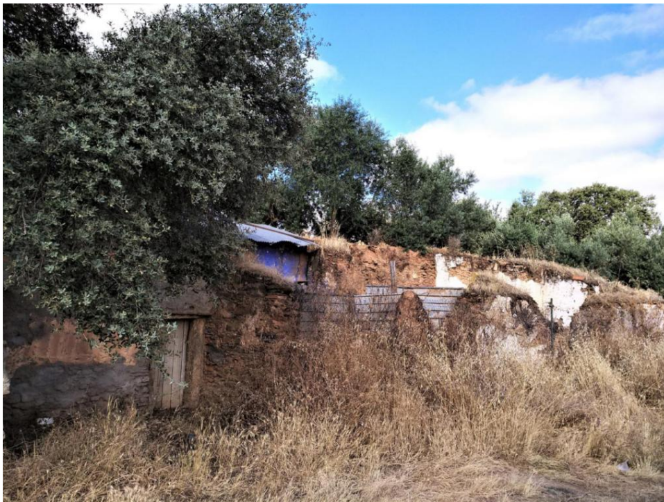
Image 192: Coloured and white interior walls seen in the ruins of an earth building. Mourão, Évora, 2018.
