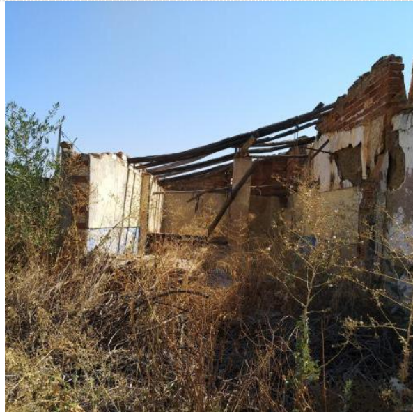
Damages incurred / problems faced: The house is in ruins, and there is vegetation inside and around it.
