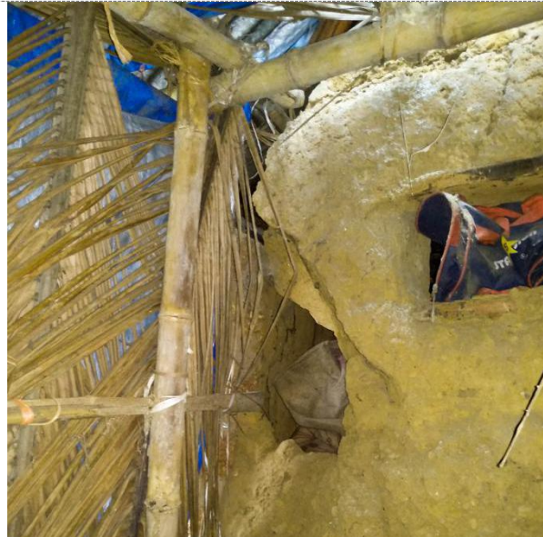
Damages incurred / problems faced: A crack in the roof caused rainwater to seep into the walls and created a hole in the corner.
