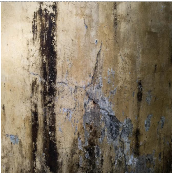
Damages incurred / problems faced: Cracks and dampness
