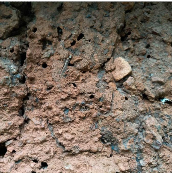
Damages incurred / problems faced: Mason-bee holes
