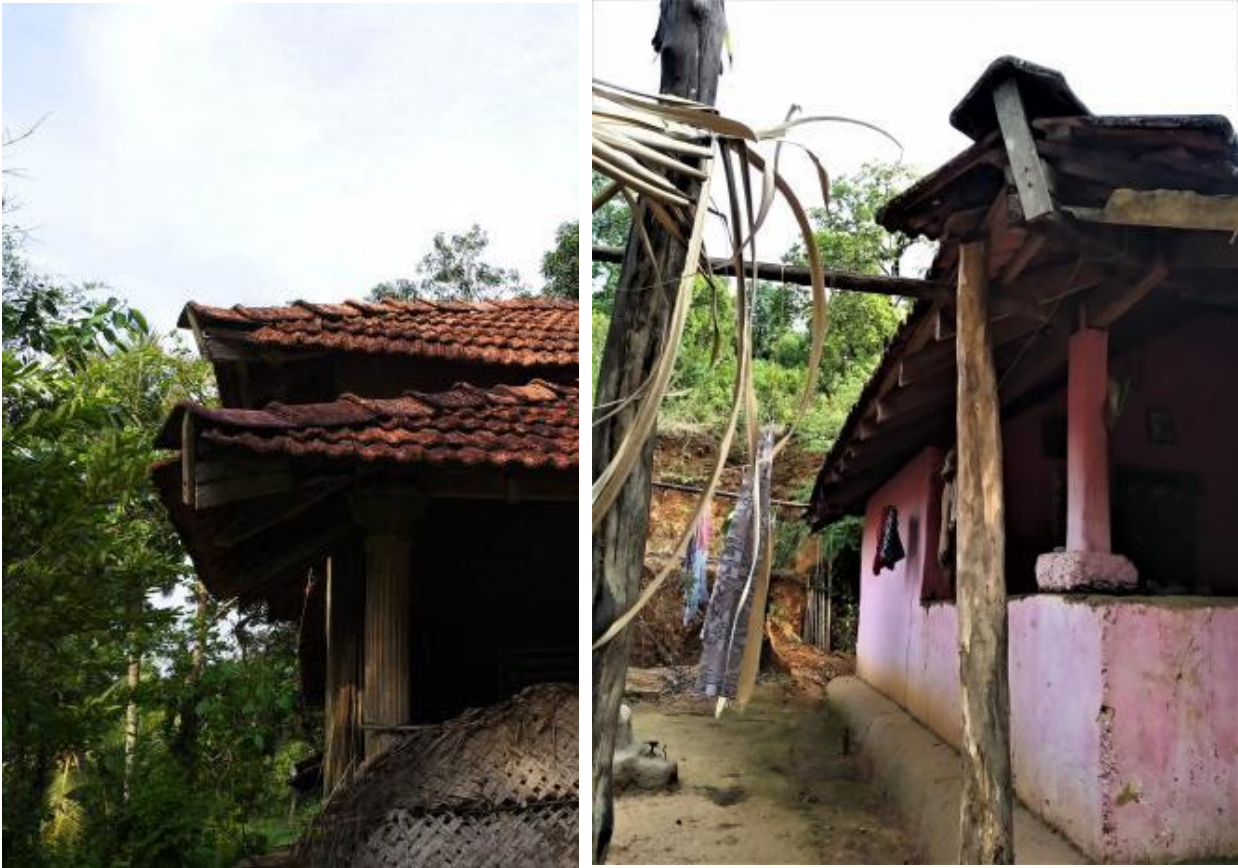
Image 129 and Image 130: Small, wooden batons were fixed on roof corners (Survey nos. 11, 13).
