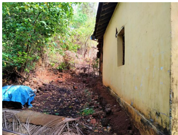
Image 89: Setback along the base-course (Survey no. 14).
