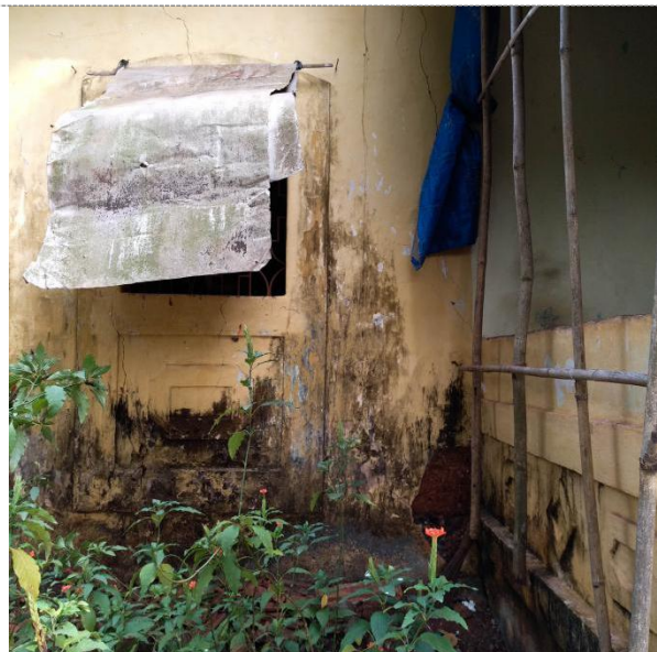
Maintenance and repairs: A make-shift overhang covers the window on the front facade.
