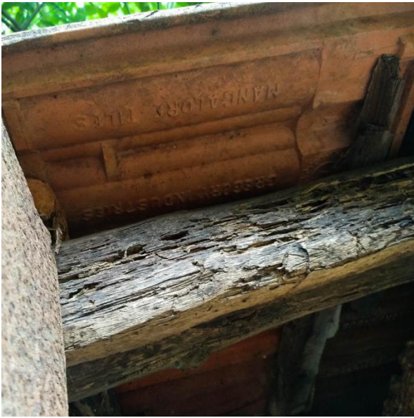
Damages incurred / problems faced: Roof-frame is rotting.
