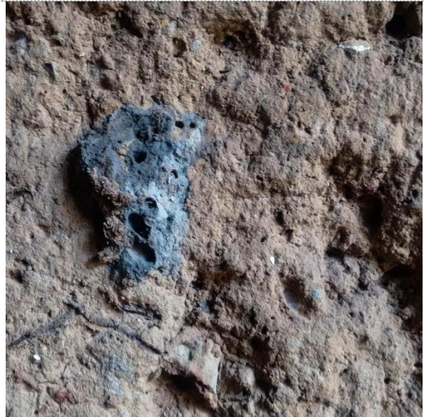
Damages incurred / problems faced: Insects have built earthen-nests on wall.
