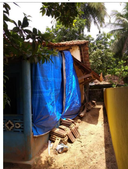
Maintenance and repairs: Tarpaulins covers are usually mounted before the monsoons and removed after the monsoons.
