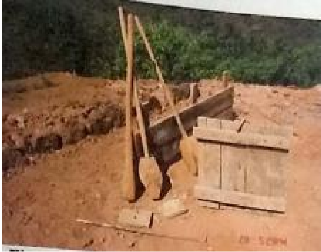
Form-work with bolts and spacers, and tools [Source: Lobo, Earth in Architecture , p.44]
