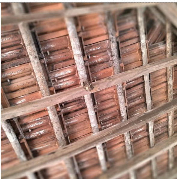
Damages incurred / problems faced: Insects called 'bateen' make nests out of mud on roofs.
