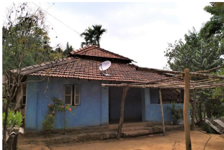
Image 109: The upper part of the roof thrusts upwards, and is separate from the lower part (Survey no. 12).
