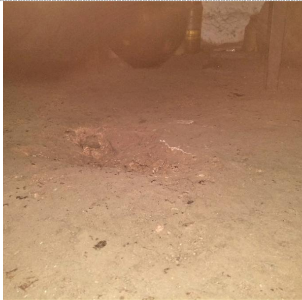
Damages incurred / problems faced: Holes and chipping on flooring.
