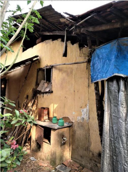
North facade, adobe-brick extension. Observations: Stepped decline on the wall top. Damages: Cracks demarcating the original, earthen-walls and the new, laterite-walls.
