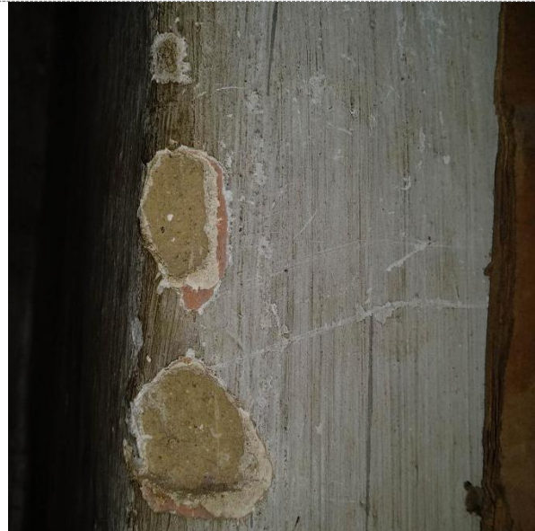
Damages incurred / problems faced: Plasters flaking and falling-off.
