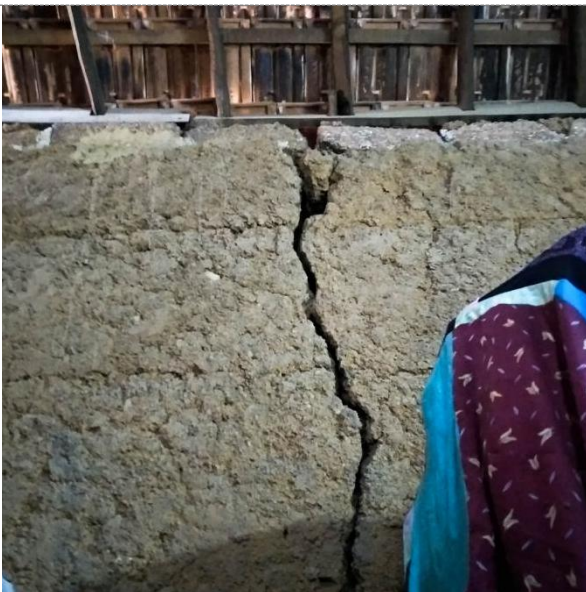
Damages incurred / problems faced: Cracks.
