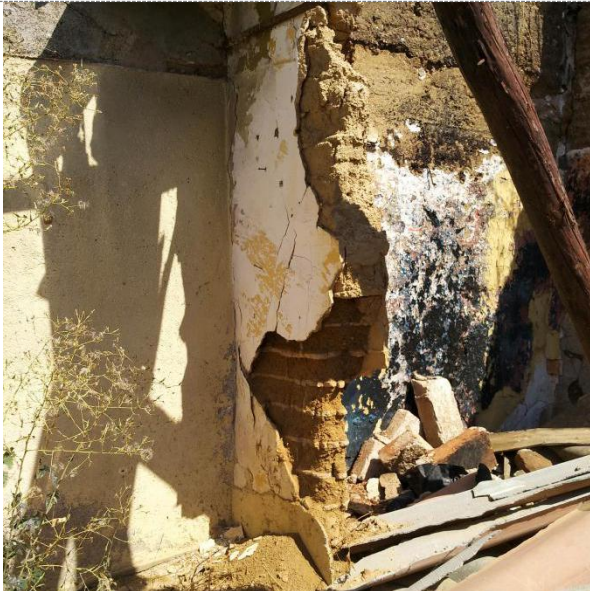
Distinct characteristics: There is an dividing wall, probably in adobe-bricks in the original building.
