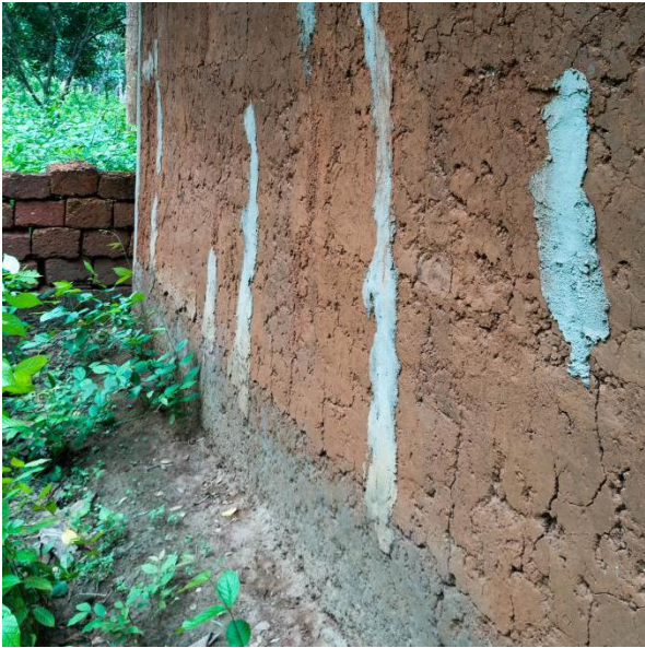
Observations: Base-course is greyish along the one facade. Repairs: Cracks and other repairs done in cement.
