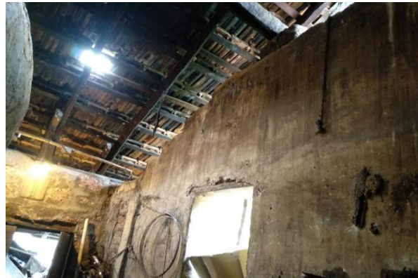
Restorations and/or interventions: The rear adobe-brick wall was torn-down and a laterite-and-cement was built in its place. Damages incurred: Walls have blackened due to the smoke from the oven.
