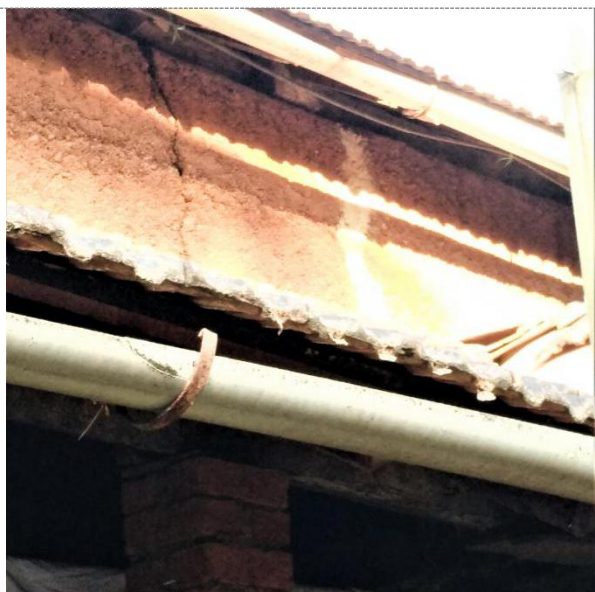
Damages incurred / problems faced: Cracks.
