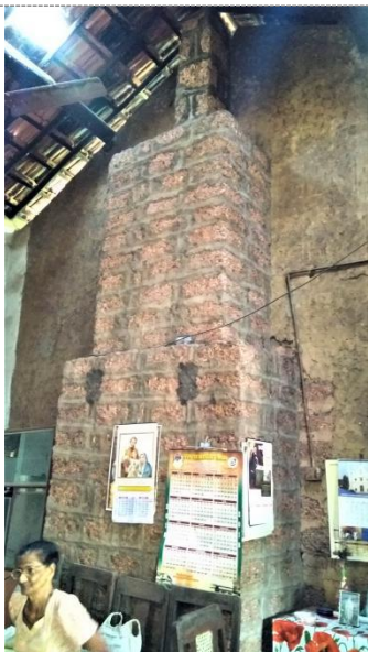
Maintenance and repairs: A laterite block was built to cover the major crack and window opening, and thereby stabilise the wall. The block turned out to be more voluminous than needed.
