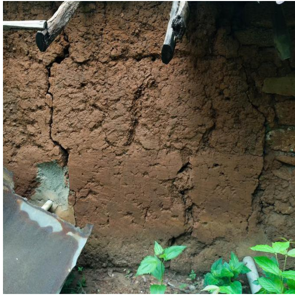
Observations: Some parts of the wall are less eroded than the others.
