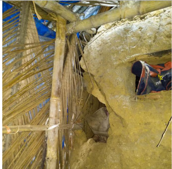
Damages incurred / problems faced: A crack in the roof caused rainwater to seep into the walls and created a hole in the corner.
