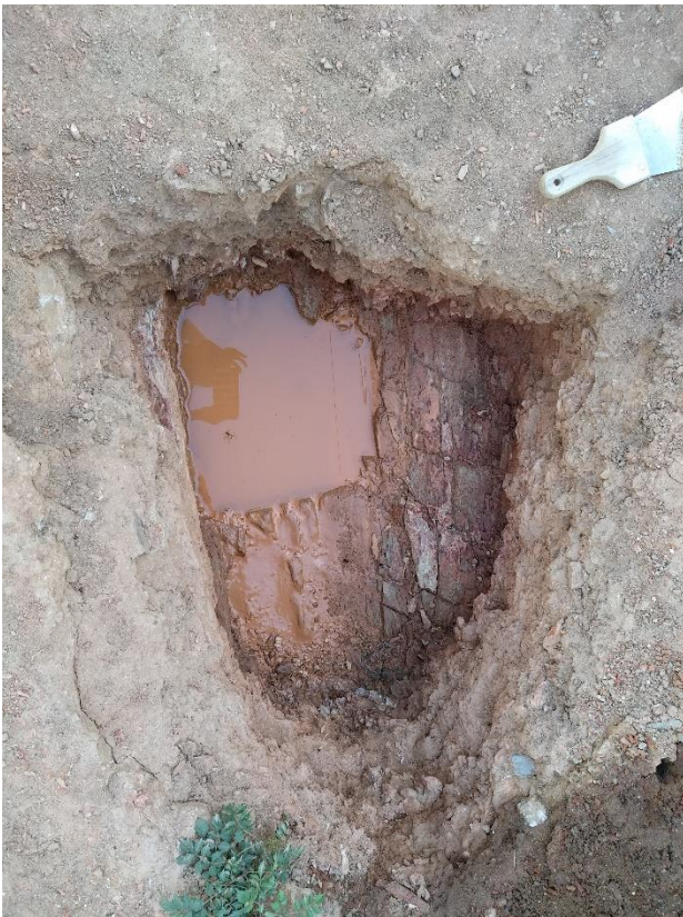
← Digging the ground in Mourão to find the depth at which the rocky ground is found. This depth determines the depth of the foundation and is likely to differ from area to area, even within the same village. (Picture taken in August 2018)
