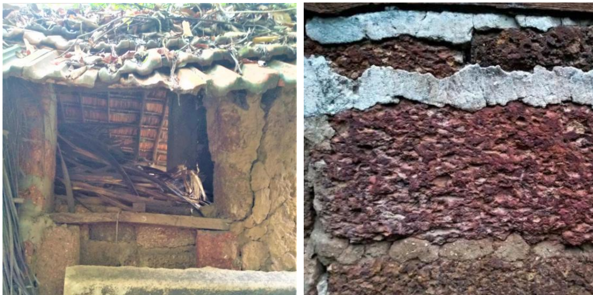
Image 134: Mortars were present in those parts of the walls that had laterite-stone masonry i.e. in the base-courses, window frames, corners, etc. (Survey no. 5).
