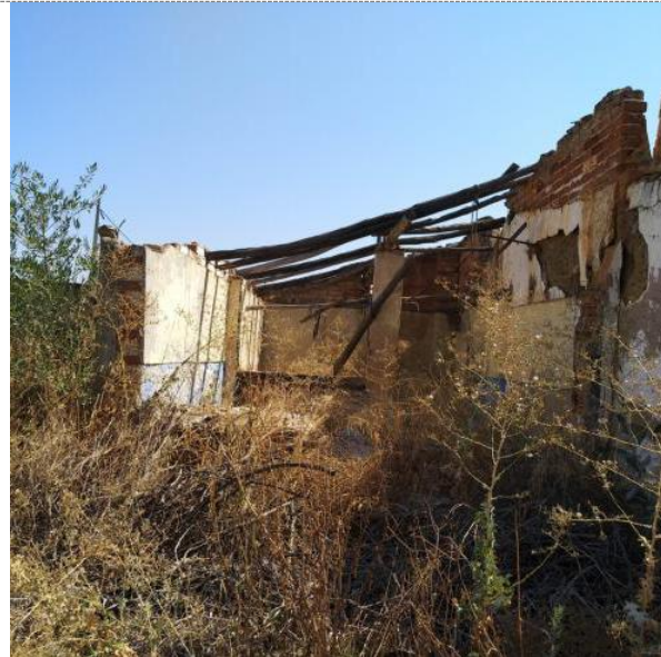
Damages incurred / problems faced: The house is in ruins, and there is vegetation inside and around it.
