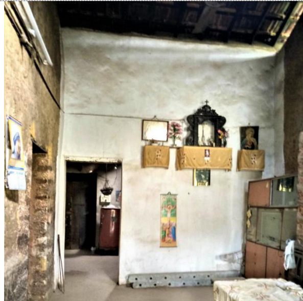
Plasters: No plaster, except kitchen and one wall in the hall are plastered with cement (interior).
