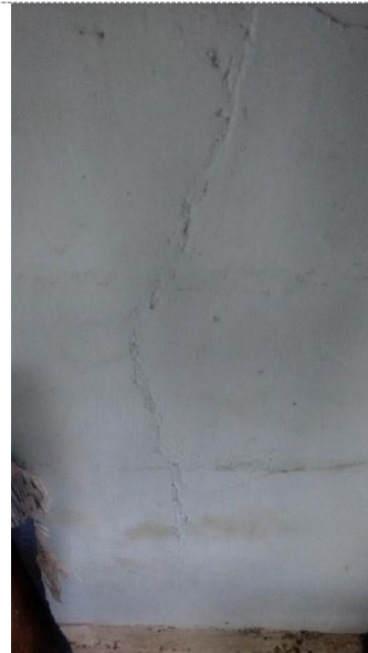
Damages incurred / problems faced: Cracks on internal walls.
