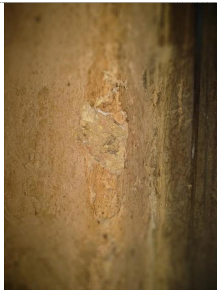
Damages incurred / problems faced: Chipping of wall edges.
