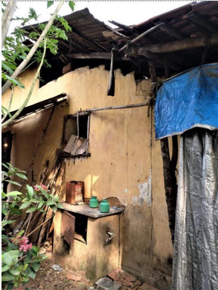
North facade, adobe-brick extension. Observations: Stepped decline on the wall top. Damages: Cracks demarcating the original, earthen-walls and the new, laterite-walls.
