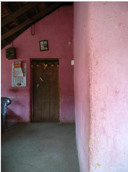
Damages incurred / problems faced: Bulging of wall.
