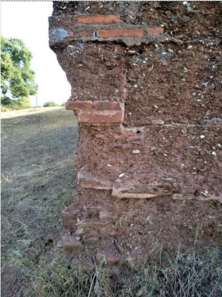
Base-course: 0.30m; in stone. Corners: In rammed-earth and fired-bricks. Distinct characteristics: Evidence of schist between the rammed-earth 'lifts'.
