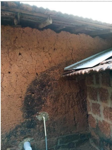
Damages incurred / problems faced: Black dampness blotch on rear wall.
