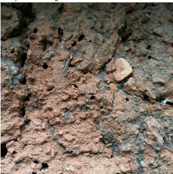
Damages incurred / problems faced: Mason-bee holes
