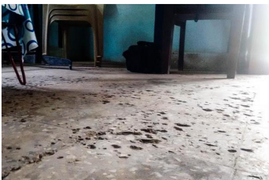
Damages incurred / problems faced: Chip-tiles are chipped-off.
