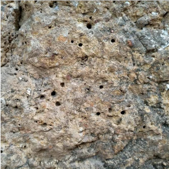
Damages incurred / problems faced: Mason-bee holes.
