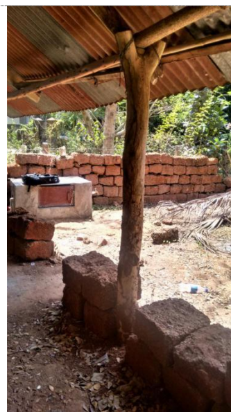
Observations: A make-shift lean-to aids in protecting facade walls from rain water. Simple branches are used to support the roof of the lean-to.
