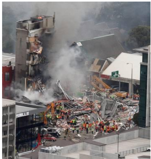
Photo 2: CTV building - Christchurch 2011 Source: Mark Mitchell
