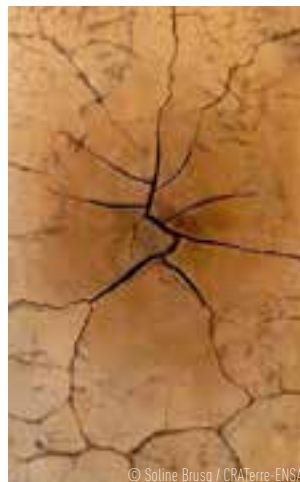
© Soline Brusq / CRATERRE-ENSAG Tableau de fissures
