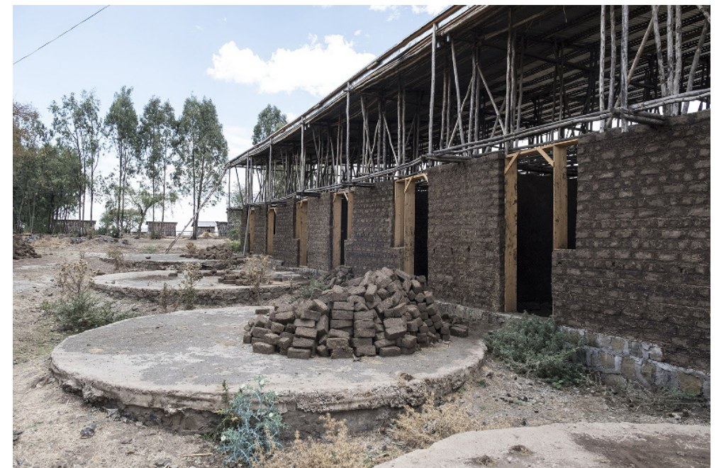
NESTown Project. Bura, Amhara. Chantier en cours de construction. Photo de NESTown.
