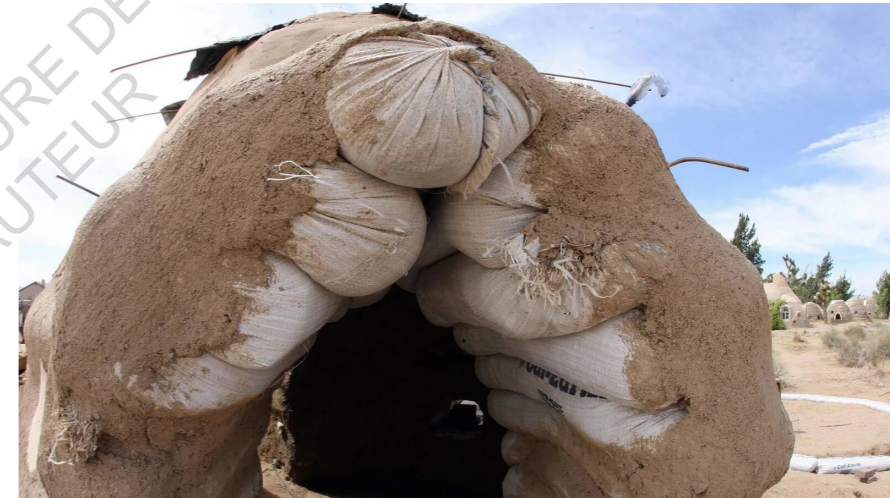
Superadobe-filled bags being covered with another earth mixture, next to finished superadobe houses at the Cal-Earth Institute
