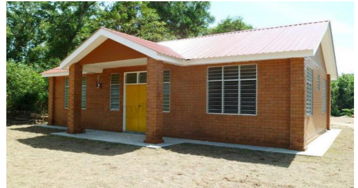
A Malaysian Interlocking Bricks column being reinforcement by steel bars and a completed public housing.
