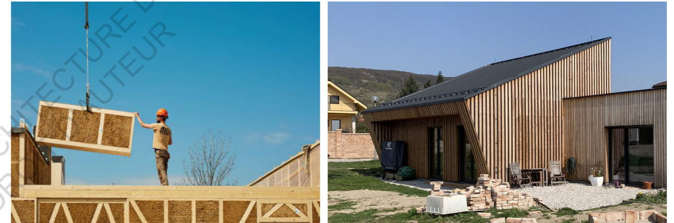
EcoCocon panel being assembled and a completed project, the Solar Kit House.
