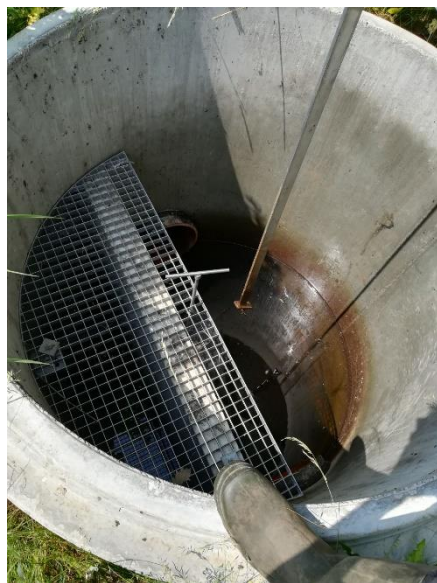
Subsurface drainage system leading to the woodchip bioreactor
