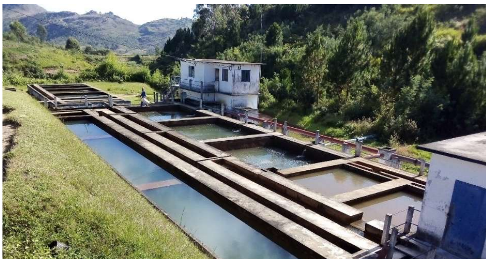
Figure 19: Photo de la station de Vatosola
