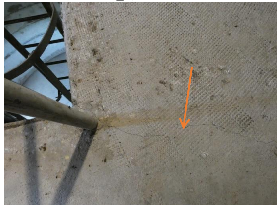
Fissuration (Fint_3) – palier P3
