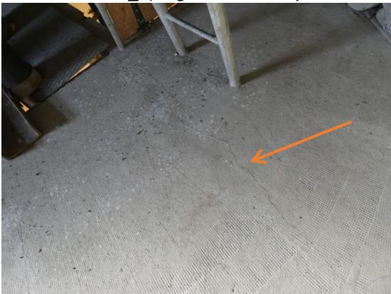
Fissuration (Fint_1) – palier P1
